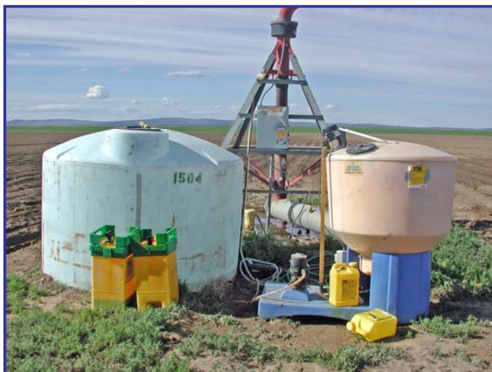
Figure 6. Identification information must appear on all application tanks, regardless of the size and content(s).
